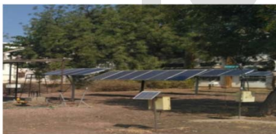
Fig.2 Solar panel installed in the energy park
